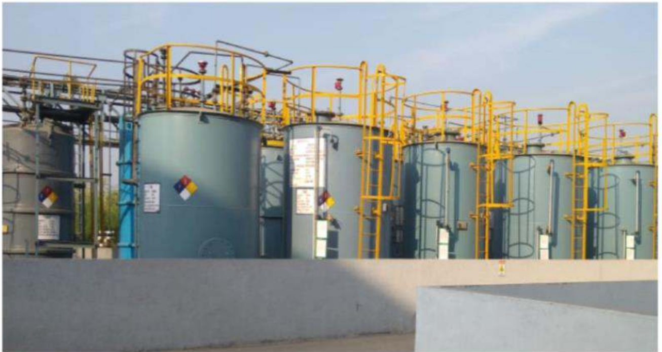
Breather Valves & Flame Arresters installed on Each Tank
