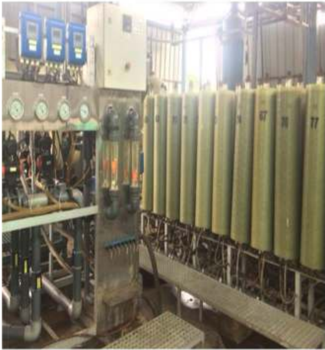
Reverse Osmosis Plant
