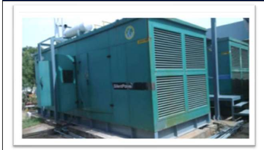
Acoustic Enclosures of DG Set
