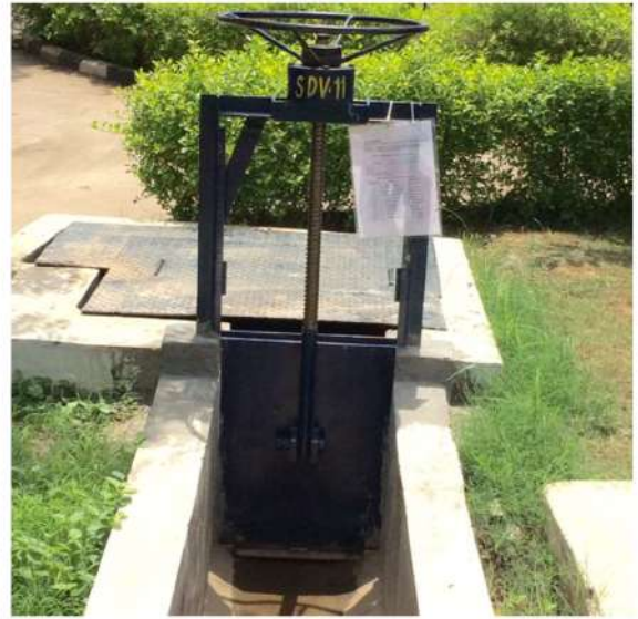
Sluice Valve at Strategic locations in storm drain
