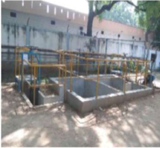
Guard Pond for Storm Drain
